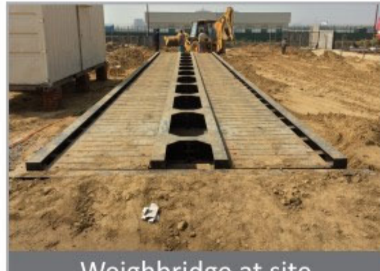
Weighbridge at site
